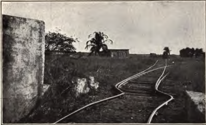
A. Subsidence of the ground with consequent tilting of buildings in the Victoria Battery, Port Royal. The kink in the railway track is over a fault.
